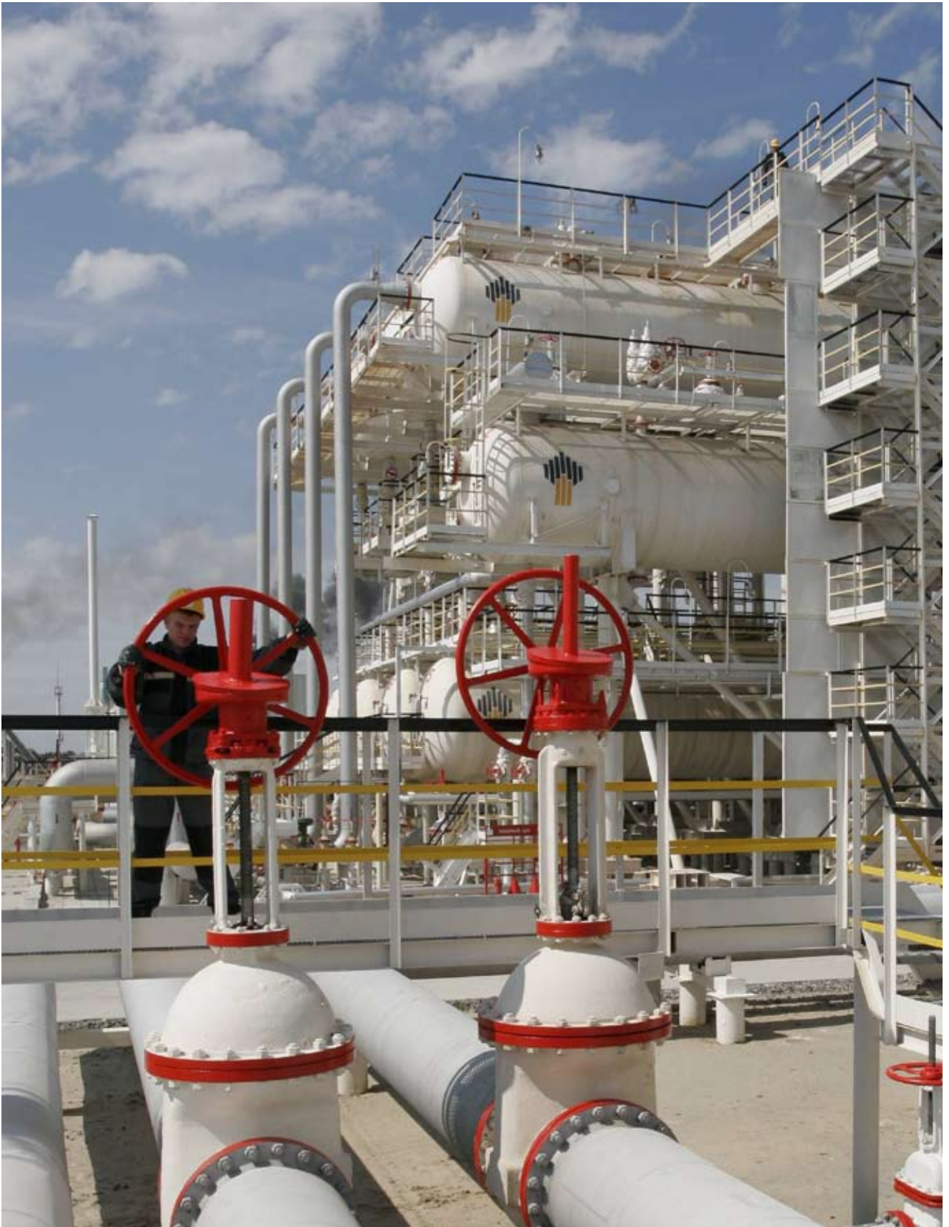
Separation unit at Central Treatment Facility – 8, Yuganskneftegaz
