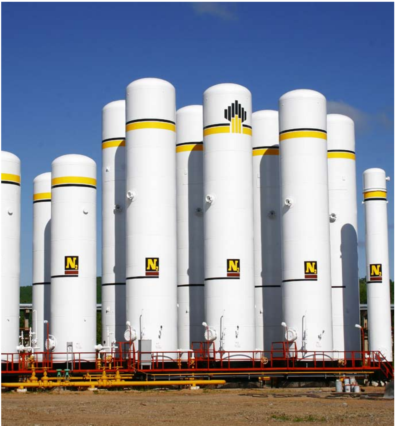
Nitrogen/oxygen unit of the Komsomolsk Refinery
